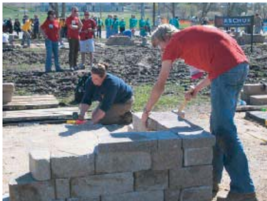
Laura McCaul, NPD '12 and Ryan Fousert, third year student work on completion of paver and stone wall installation.
